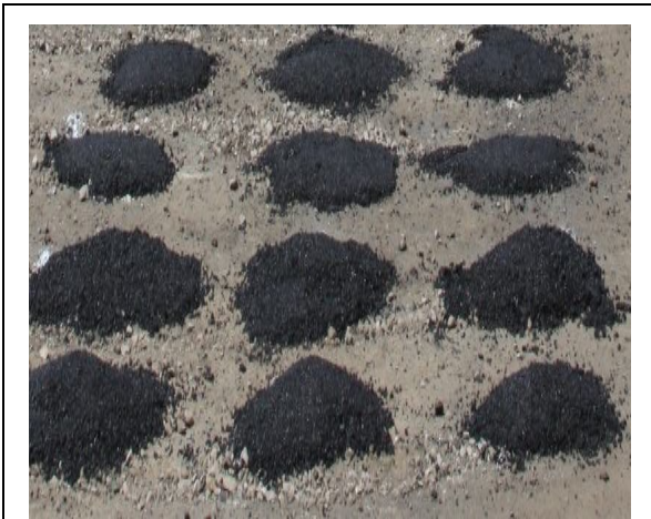
Fig. 5. The gages covered with the #4 sieved asphalt mixtures just before paving over the sensors area. The mixture was hand compacted with tamping rod as best as possible without damaging the sensors.
